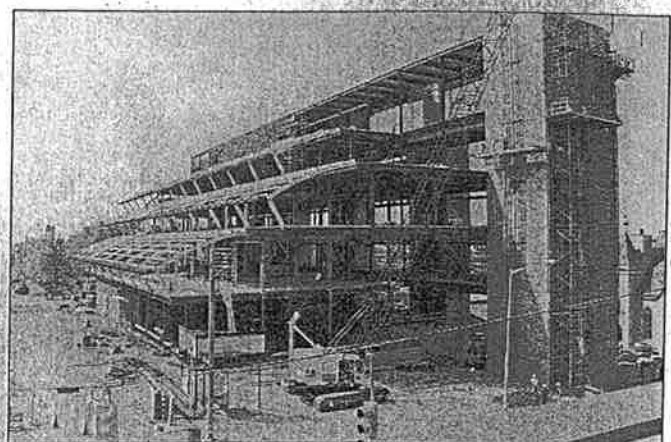
The view looking northeast shows work underway on the facility and its major tower structures.
