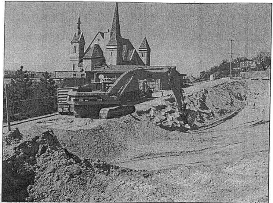
Dykema Excavating of Grand Rapids uses their model 330 Cat backhoe fitted with a 1-1/2-cubic-yard bucket to begin excavation for the new, $200-million Van Andel Institute building.
