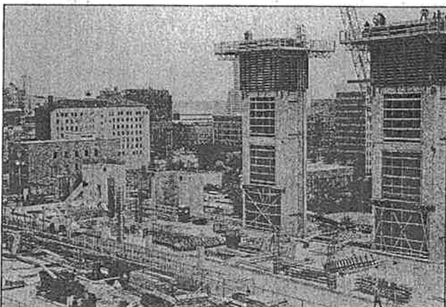
Erhardt's 75-ton P&H crane at work on one of the two major towers that will anchor the interior of the facility.
