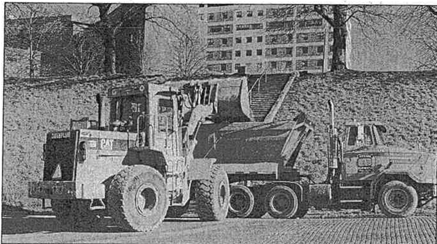
A model 950F Cat front end loader handles a 2-1/2-cubic-yard bucket for Dykema Excavating in loading out broken concrete on the project. (Note: Part of Spectrum Hospital is seen in the upper background).
